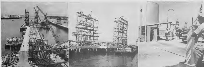
STRUCTURES FOR free-standing loading arms and the arms themselves have been erected on Lago's No. 3 Finger Pier. The new pier virtually looks as it will when fully completed. Most piping, left, has been installed out to the breasting island. Free-standing loading arms on the two structures, center, have been undergoing tests. The project sparked remote-control gates, right, at gate No. 2. The guards will also operate gates to the pier access road.
